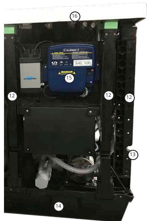
Corner Compartment (left front)
